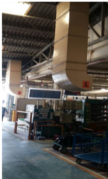
Set up ventilation system for heat reduction
